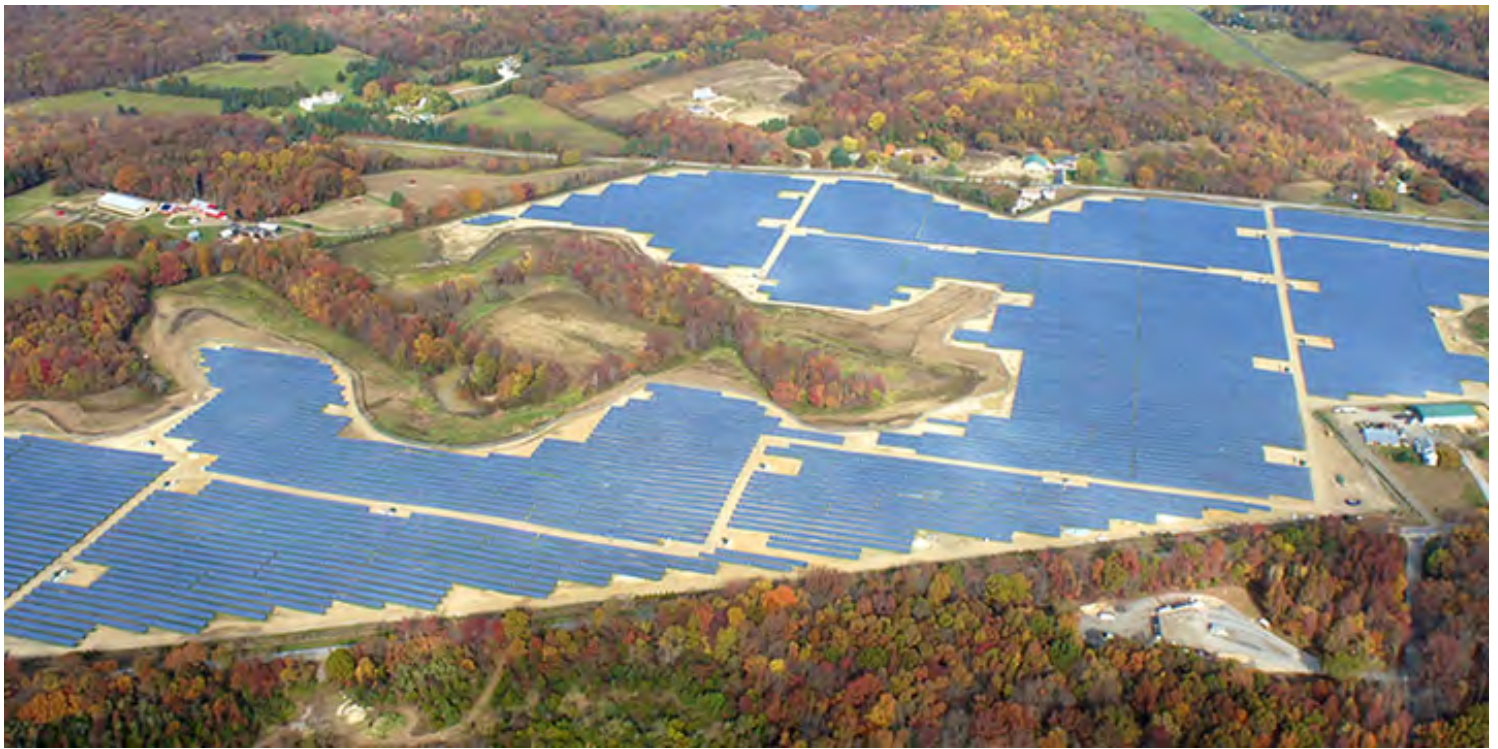
Con Edison Development's solar farm in Pilesgrove, New Jersey, is helping to reduce carbon emissions.
